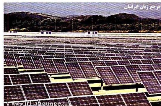
A field of solar panels
