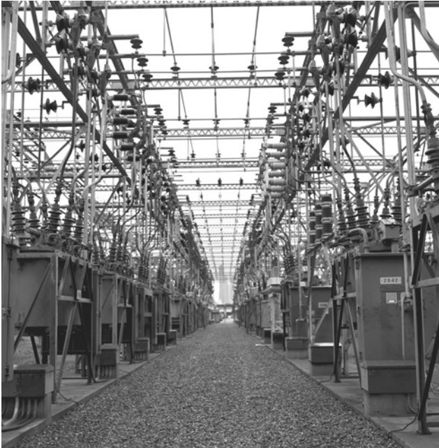
Figure 5-1 Distribution substation. Reproduced with permission of Fotosearch.
