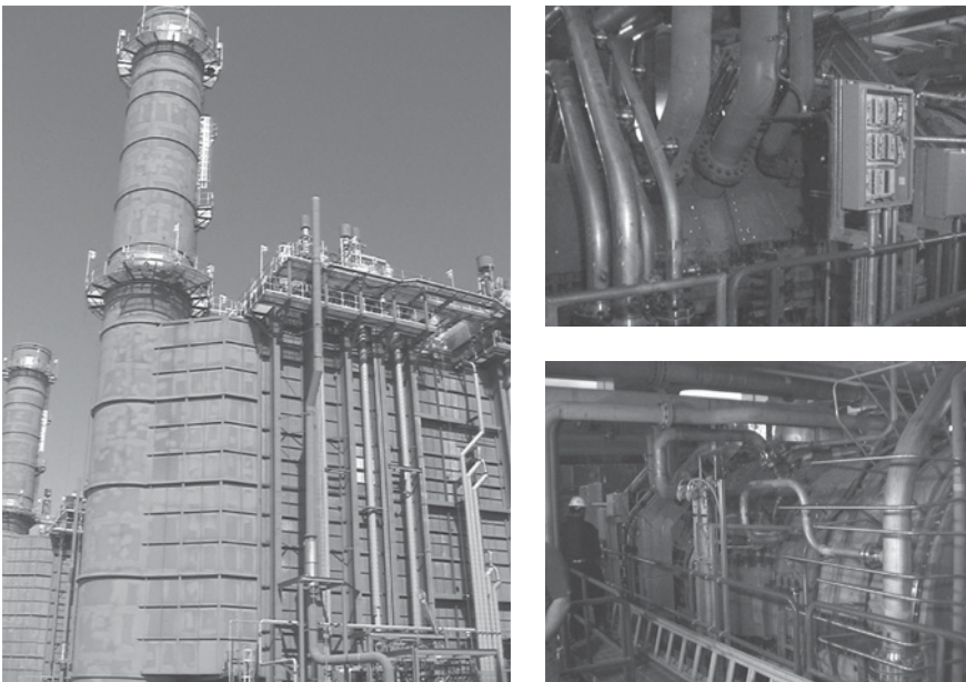
Figure 2-10 Combined cycle power plant.
