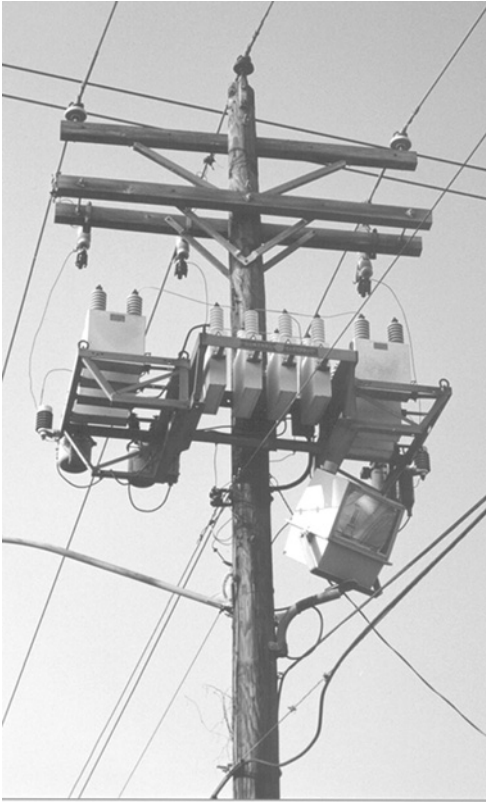
Figure 4-42 Distribution capacitor bank.
