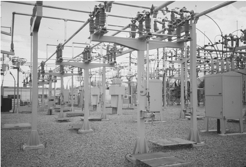
Figure 4-40 Example of typical electrical bus.
