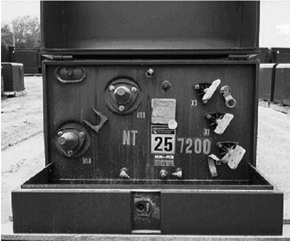
Figure 5-34 Switching transformer. Courtesy of Alliant Energy.
