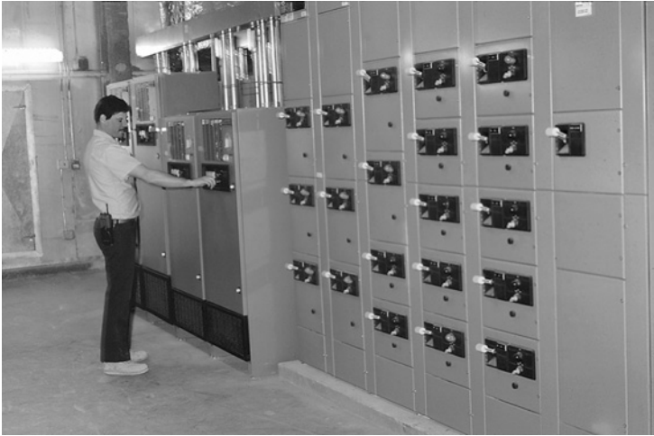
Figure 6-21 Industrial panel. Reproduced with permission of Photovault.
