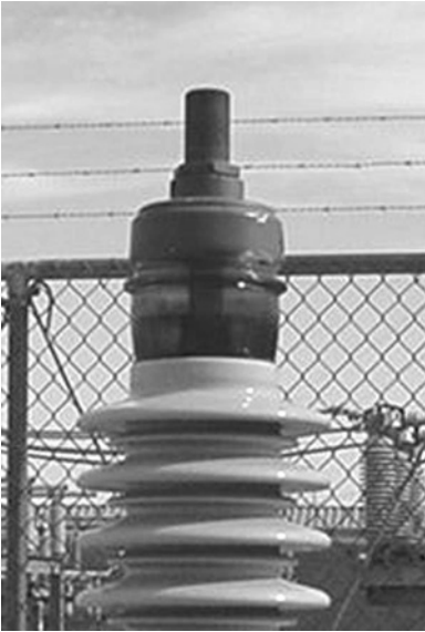
Figure 4-7 Bushing oil level gauge.
