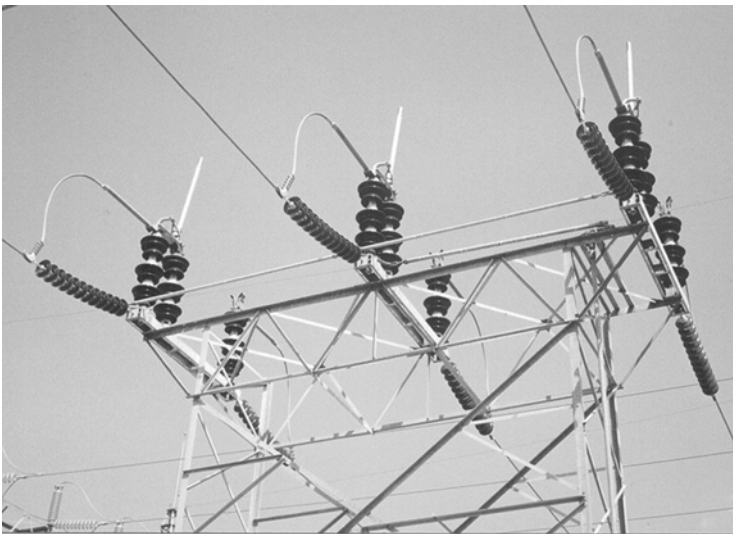
Figure 4-34 Vertical break. Courtesy of Alliant Energy.
