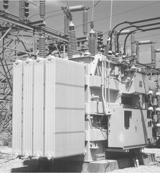
Figure 4-2 Distribution power transformer.
