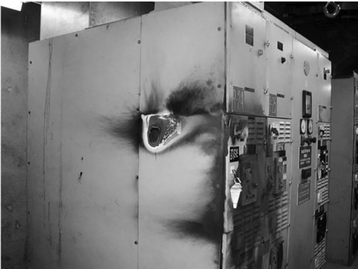
Figure 10-13 Arc-flash. Reproduced with permission of from LSelectric.
