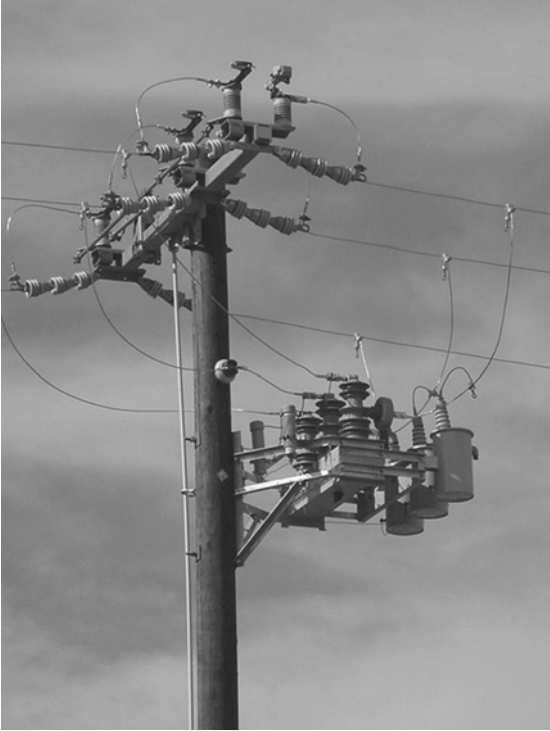
Figure 6-12 Overhead primary metering.
