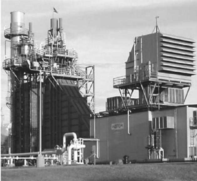
Figure 2-9 Combustion turbine power plant.
