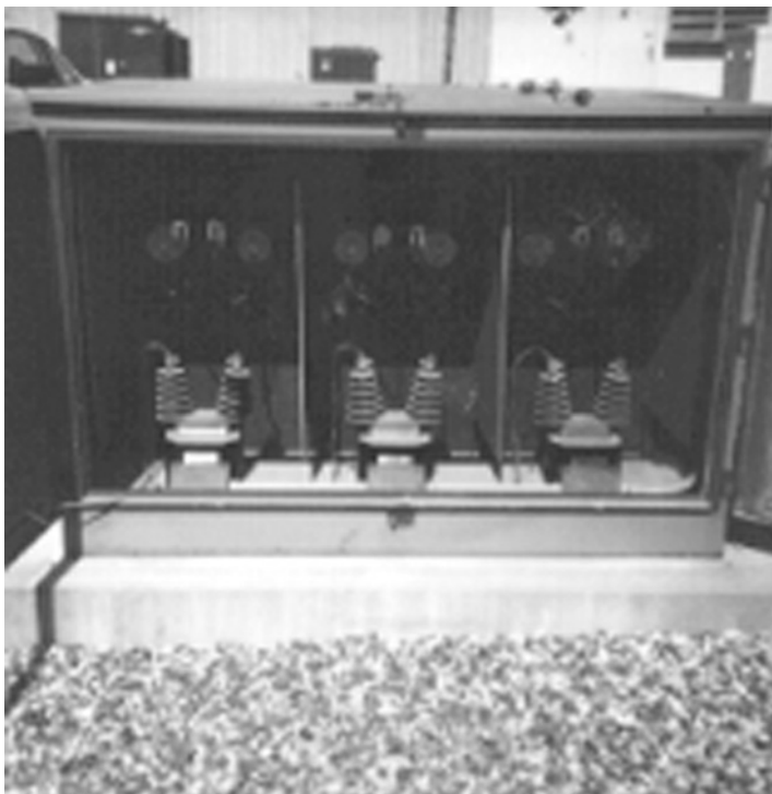
Figure 6-11 Underground primary metering. Courtesy of Alliant Energy.
