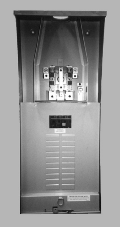
Figure 6-14 Meter cover removed.
