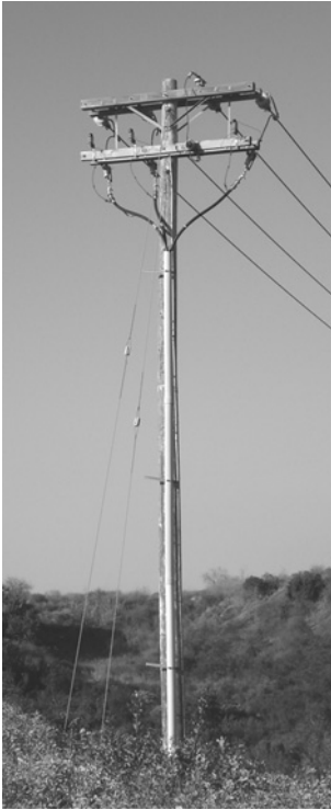
Figure 5-27 Dip pole or riser pole.
