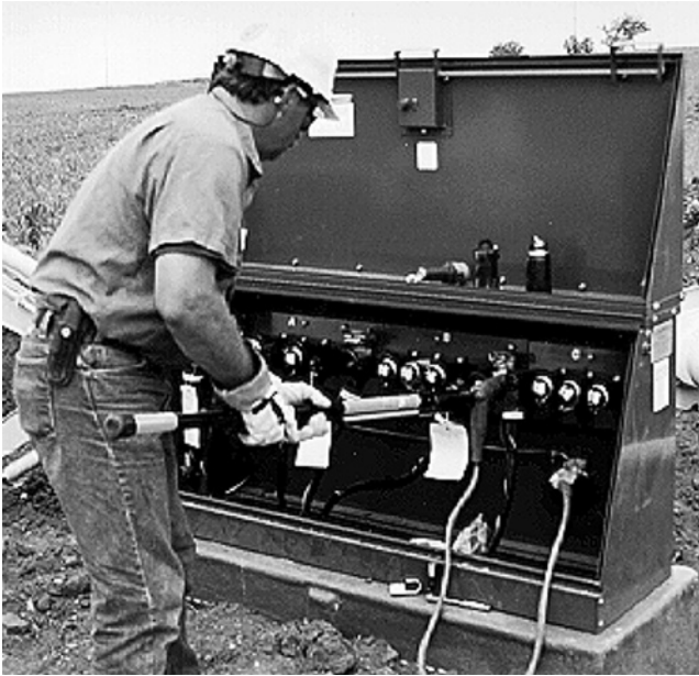
Figure 5-29 Load break connections. Courtesy of Alliant Energy.
