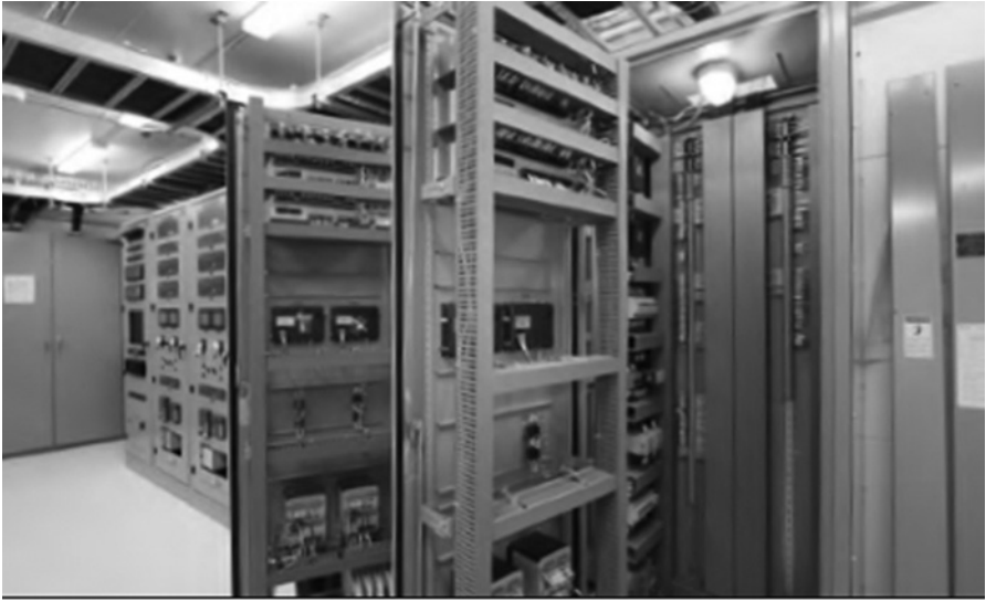
Figure 4-46 Control building. Courtesy of Schweitzer Engineering Laboratories, Inc.
