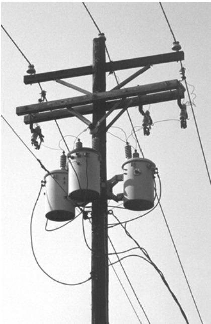
Figure 5-18 Three-phase transformer bank.
