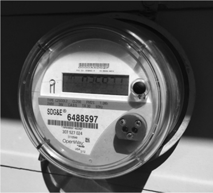
Figure 6-9 Residential smart meter.
