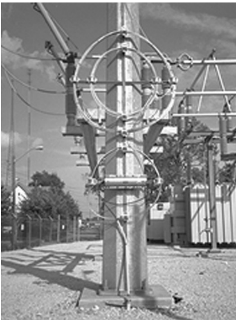
Figure 9-6 Substation fiber optics.
