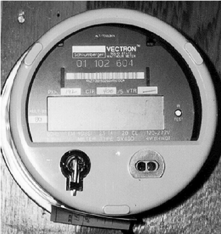
Figure 6-6 Solid-state kWh meter.
