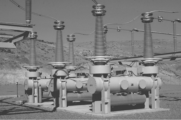
Figure 4-27 345 kV gas breaker.
