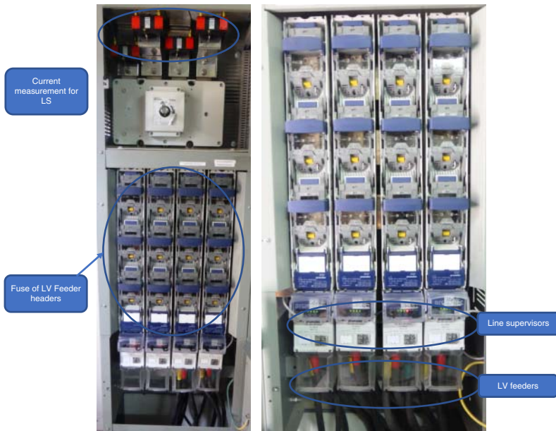
Figure 8.5 Photos of an electrical cabinet of an LV transformer station where line supervisors have been installed as a part of an advance simple entity (ASEN).
