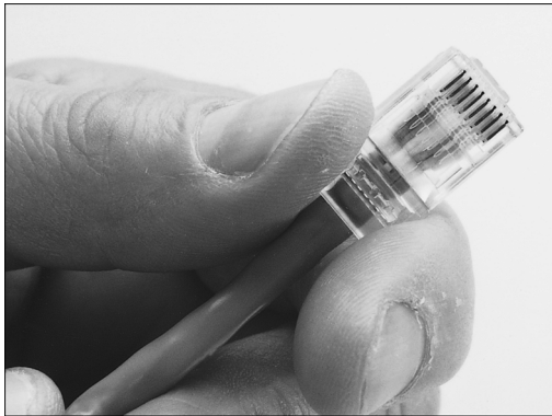
Figure 20.21 Push the RJ-45 connector into place, ensuring the cable pairs are ordered properly.
