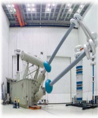
UHV DC Converter Transformer
