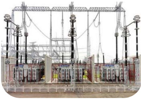
UHV AC Transformer
