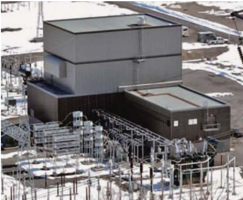
Figure A.16 Scene of the substation with the world's first VFT [7].
