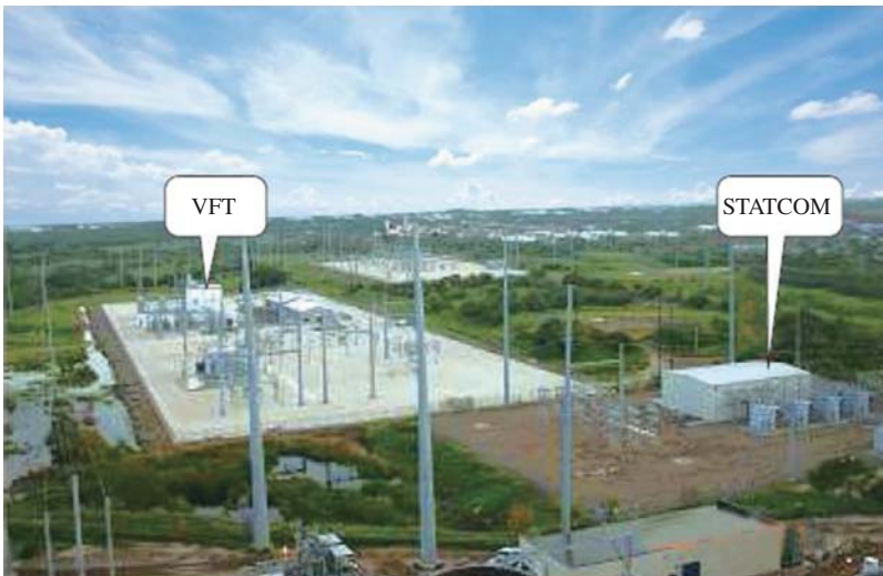
Figure A.22 Outside view of the Laredo Substation [4].
