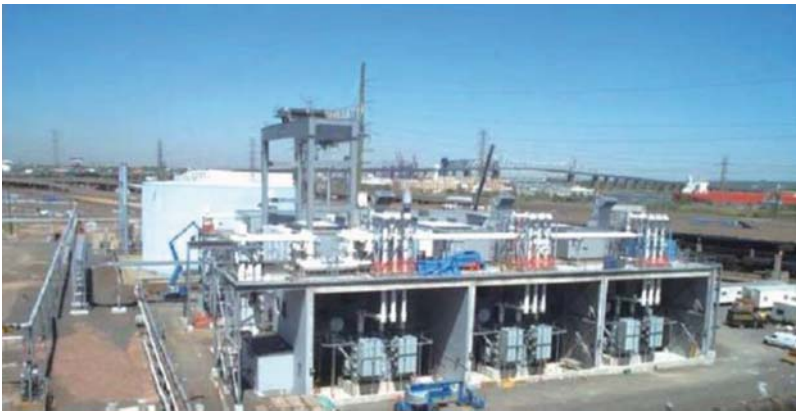
Figure A.25 Outside view of the compact Linden Substation [2].
