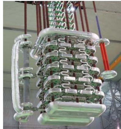
UHV DC Converter Valves
