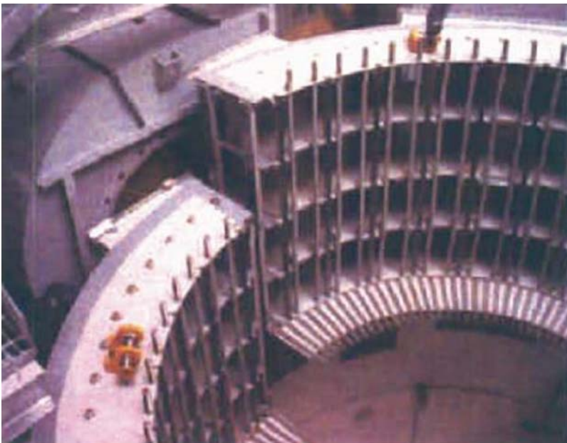
Figure A.12 Stator installation of a VFT [6].
