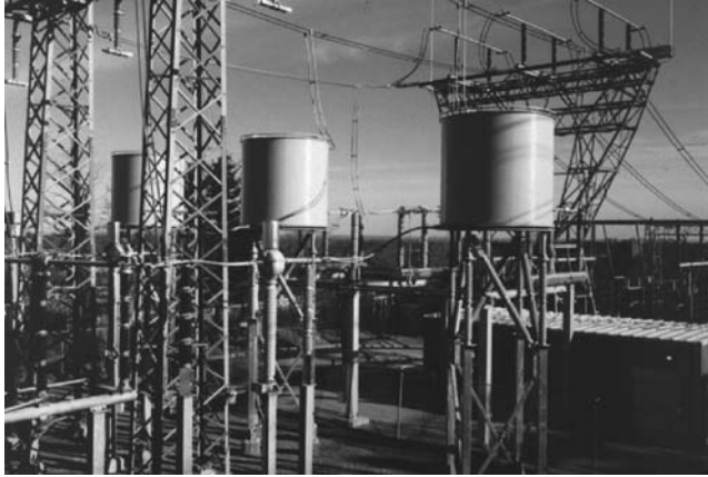
FIGURE 2.9.6 345-kV phase reactors.
