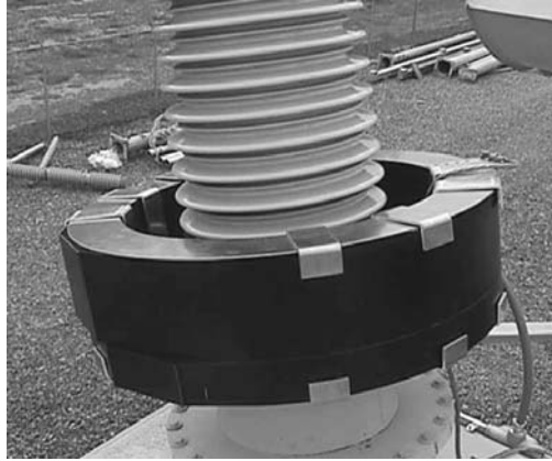
FIGURE 2.6.27 00-V-class slipover CT installed on high-voltage bushing with ground shield. Note the ground lead going back through the CT window to avoid shorted electrical turn. (Photo courtesy of Kuhlman Electric Corp.)
