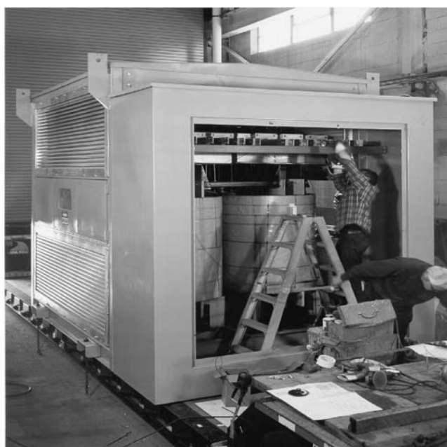
FIGURE 2.4.20 A 24-pulse dry-type transformer. 7000-kVA drive duty transformer, to be located in a tunnel, made of two 3500-kVA 12-pulse transformers. Each core and coil has 1100-V delta and wye secondary windings. Each core and coil has a 13,200-V extended-delta primary winding. One core and coil has its primary winding shifted -15^\circ , while the other core and coil has its primary winding shifted +15^\circ . One reconnectable primary spare core and coil can be used to replace either core and coil assembly. (Photo courtesy of Niagara Transformer Corp.)
