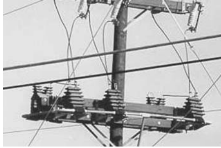
FIGURE 2.6.29 5-kV three-phase/four-wire metering rack with 3 VT and 3 CT. (Photo courtesy of Kuhlman Electric Corp.)
