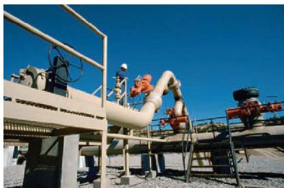
▲ Figure 10.15 A natural gas pipeline junction.
