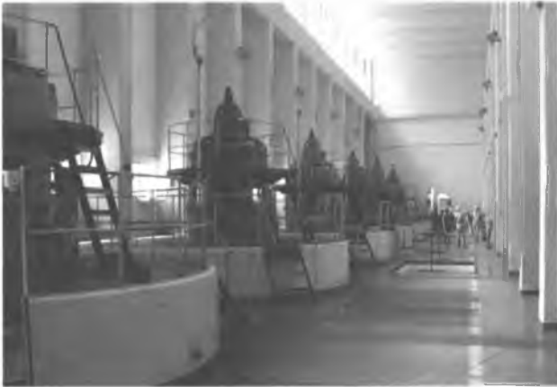
Figure 3.7. Aggregates that convert water flow into electricity in hydropower plants.
