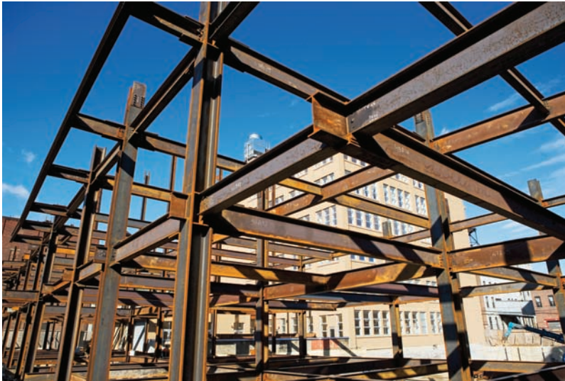
Photo 9.4 The maximum deflection of each beam supporting the floors of a building should be taken into account in the design process.
