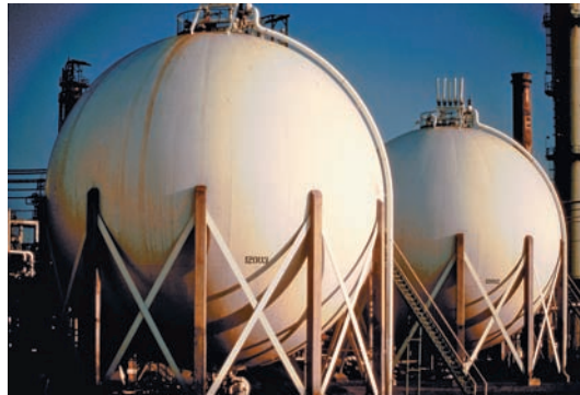
Photo 7.4 Spherical pressure vessels at a chemical plant.
