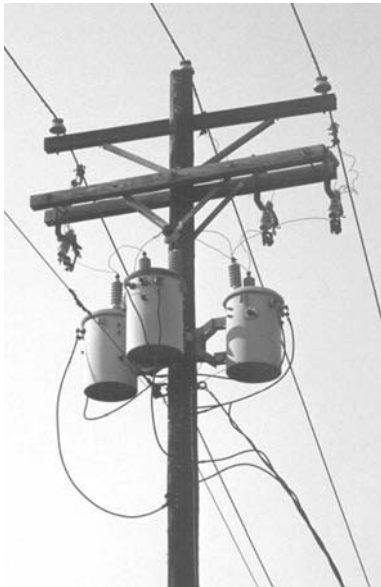
Figure 5-18. Three-phase transformer bank.
