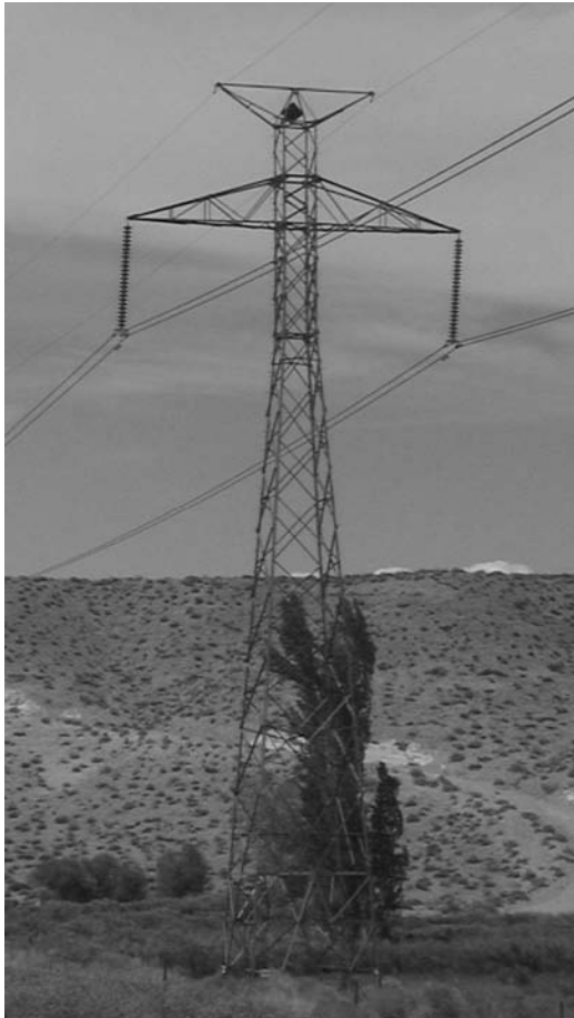
Figure 3-7. Overhead dc transmission line.
