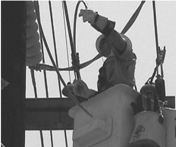
Figure 10-11. Live maintenance distribution. Courtesy of Alliant Energy.
