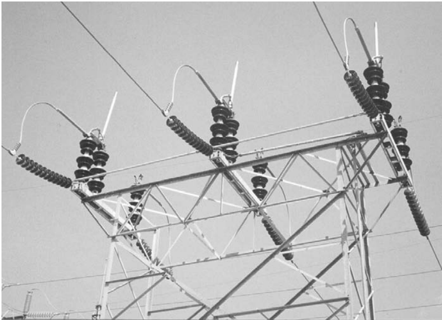
Figure 4-32. Vertical-break switch. Courtesy of Alliant Energy.
