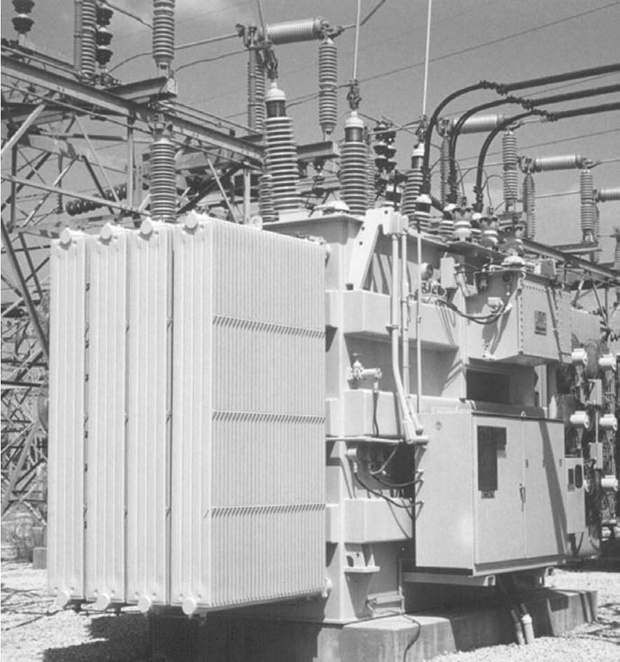
Figure 4-2. Distribution power transformer.
