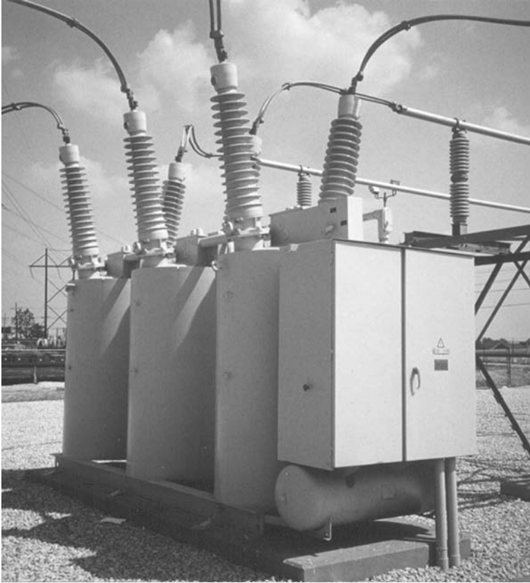
Figure 4-23. Oil circuit breaker.
