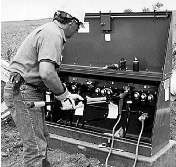
Figure 5-29. Load-break connections. Courtesy of Alliant Energy.
