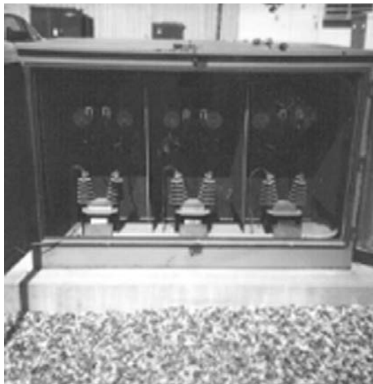
Figure 6-10. Underground primary metering. Courtesy of Alliant Energy.
