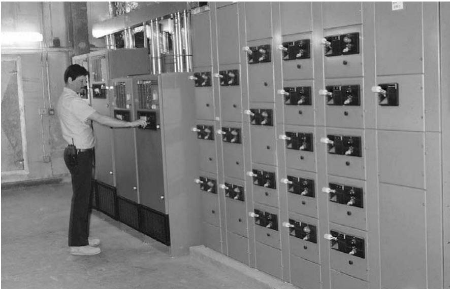
Figure 6-20. Industrial panel. Source: Photovault.
