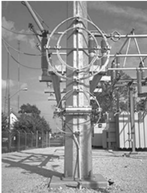
Figure 9-4. Substation fiber optics.
