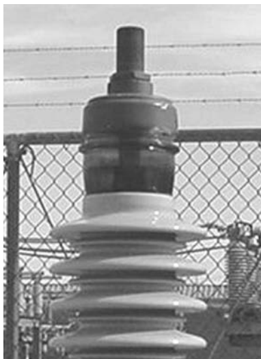
Figure 4-7. Bushing oil level gauge.
