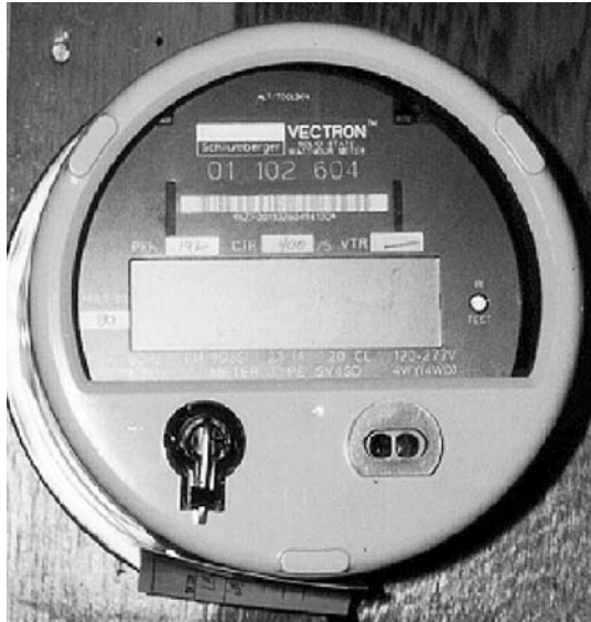
Figure 6-7. Solid-state kWh meter.
