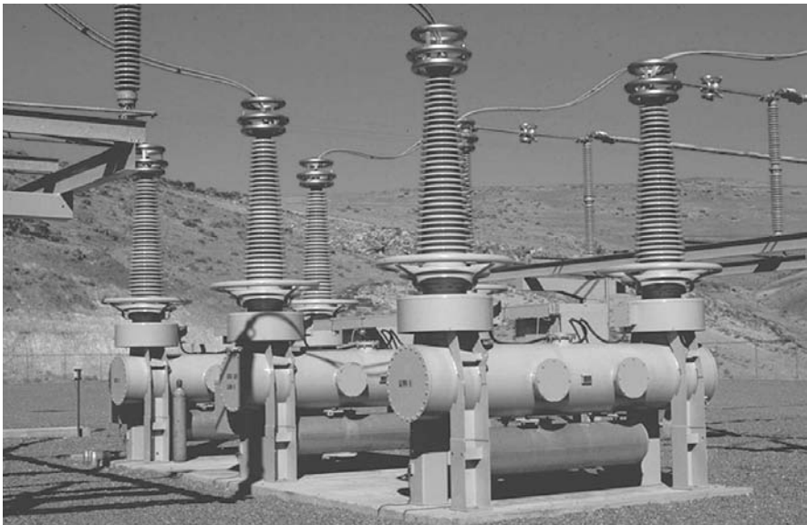
Figure 4-26. 345 kV Gas breaker.
