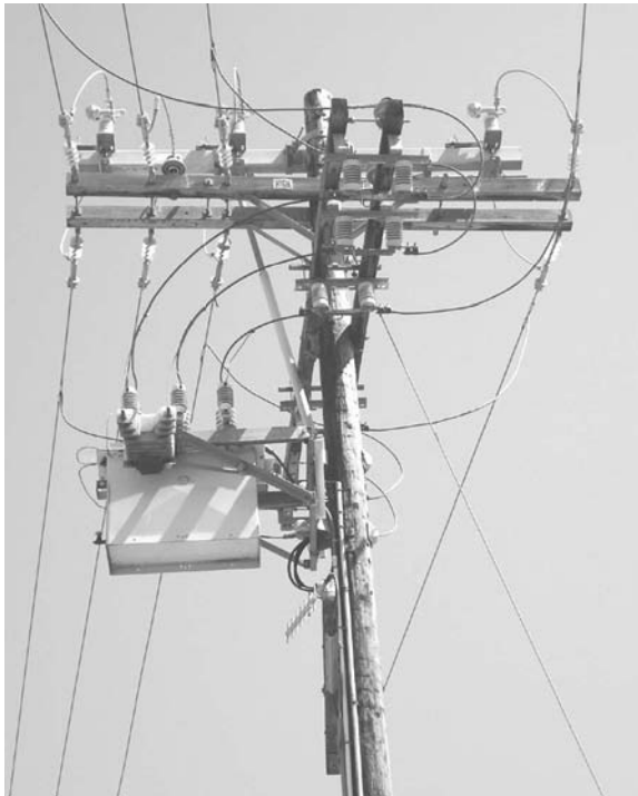
Figure 4-30. Distribution line recloser. Courtesy of Alliant Energy.
