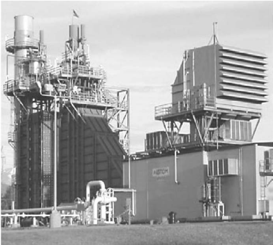
Figure 2-20. Combustion turbine power plant.
