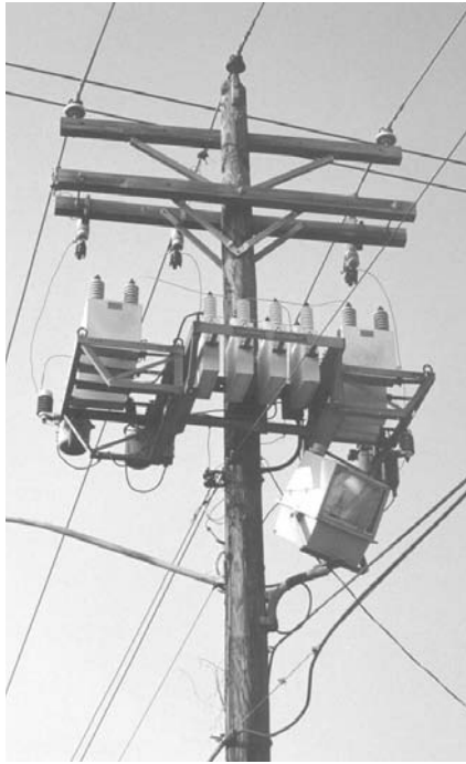
Figure 4-40. Distribution capacitor bank.
