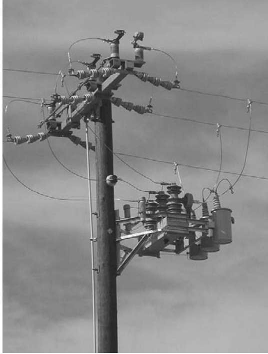
Figure 6-11. Overhead primary metering.
