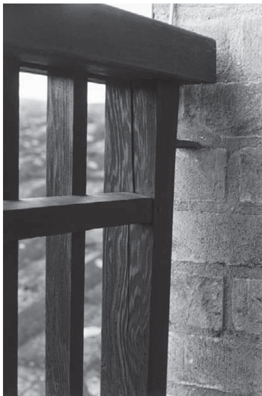
An 18-inch crack in another balustrade.
