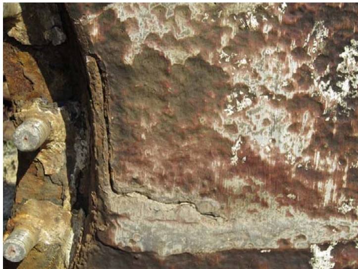
FIGURE 17.12 Fatigue crack in the deck of a ship.
