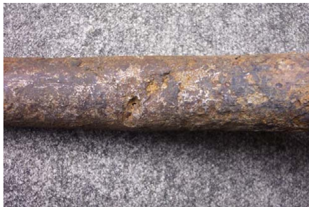
FIGURE 26.13 Pitting corrosion in an underground water pipe.
