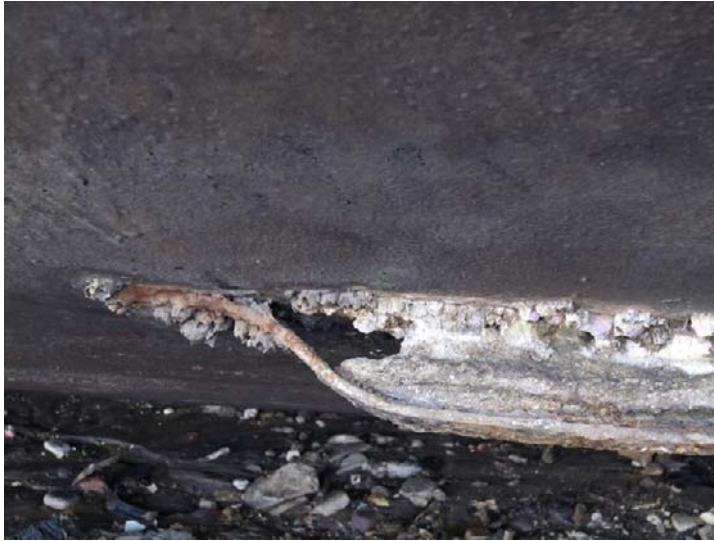
FIGURE 27.3 Magnesium sacrificial anode showing heavy corrosion of magnesium.
