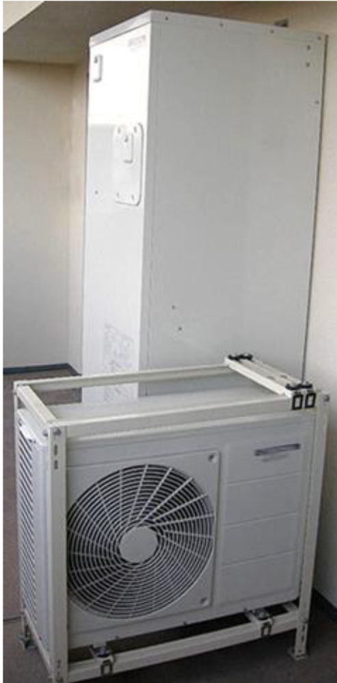
Figure 4.7 Heat pump water heater.
