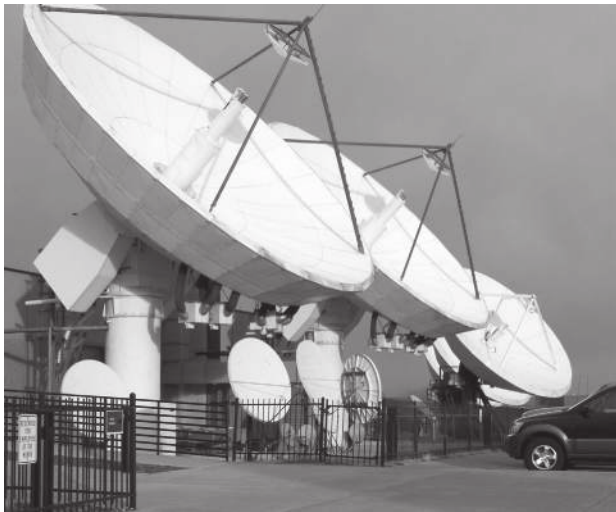
Figure I.9. A few of the several dozen transmitting antennas at EchoStar's Network's uplink facility in Cheyenne, Wyoming.
