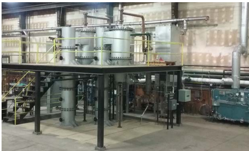
Figure 4.18 Photograph of University of Utah chemical looping PDU.
