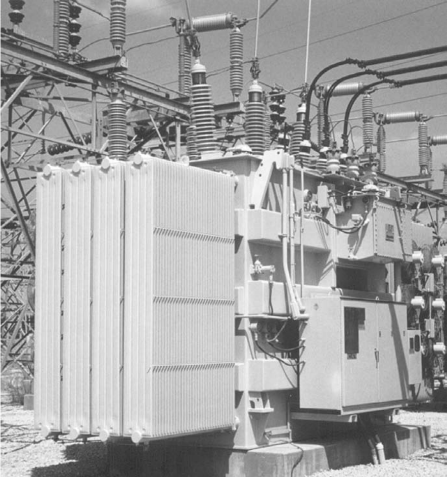
Figure 4-2. Distribution power transformer.
