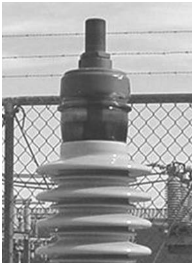
Figure 4-7. Bushing oil level gauge.
