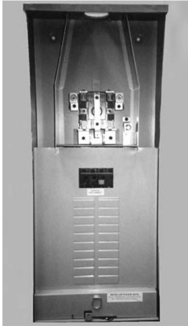
Figure 6-13. Meter cover removed.
