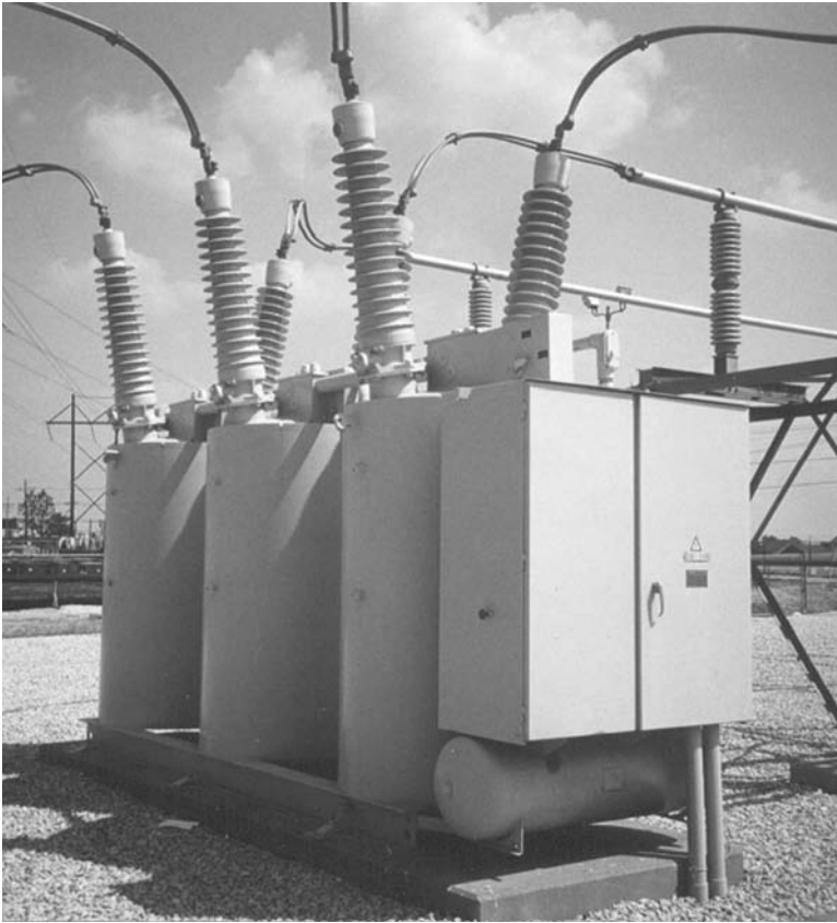
Figure 4-23. Oil circuit breaker.
