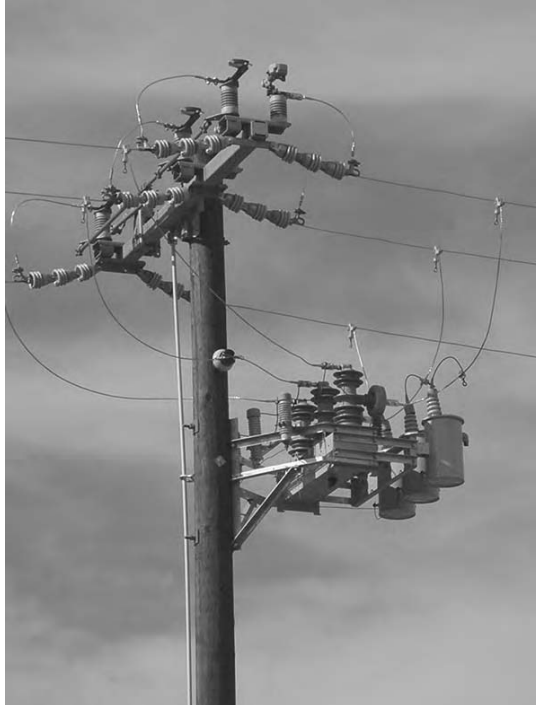
Figure 6-11. Overhead primary metering.
