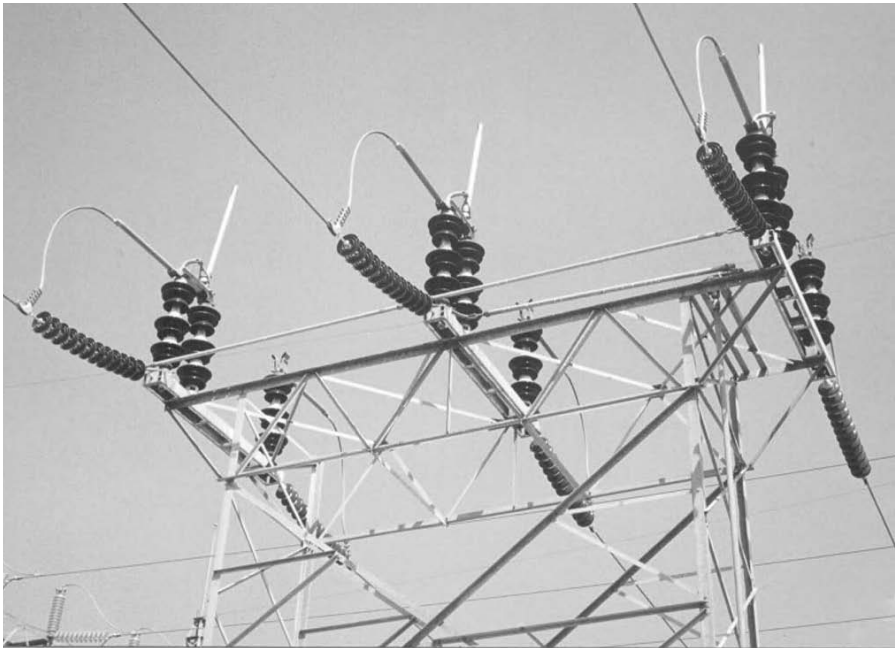
Figure 4-32. Vertical-break switch. Courtesy of Alliant Energy.
