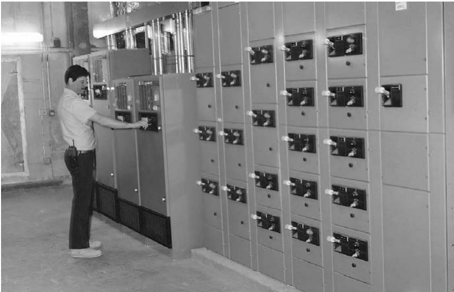
Figure 6-20. Industrial panel. Source: Photovault.
