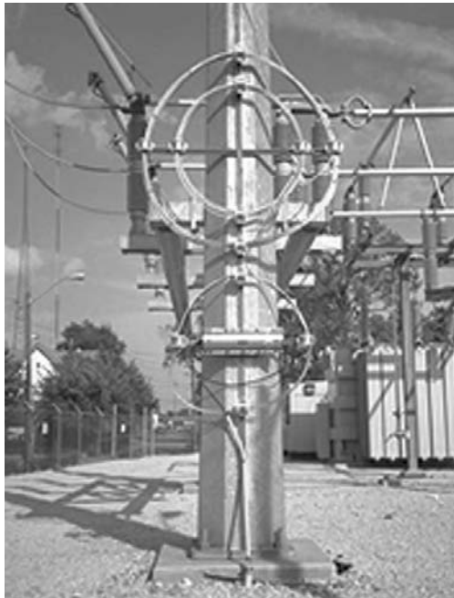
Figure 9-4. Substation fiber optics.
