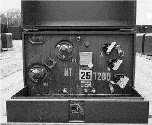
Figure 5-34. Switching transformer. Courtesy of Alliant Energy.
