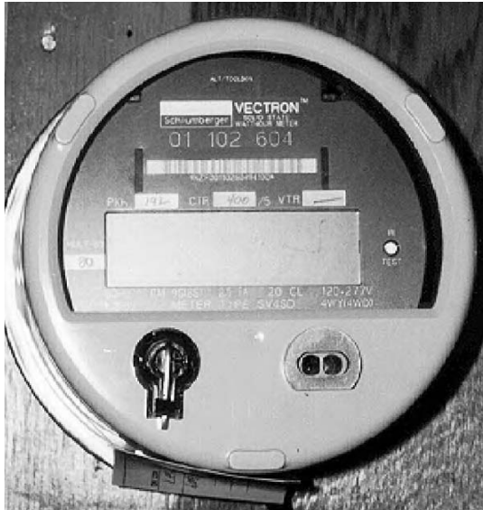
Figure 6-7. Solid-state kWh meter.
