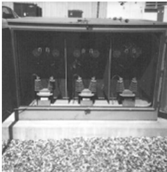
Figure 6-10. Underground primary metering. Courtesy of Alliant Energy.
