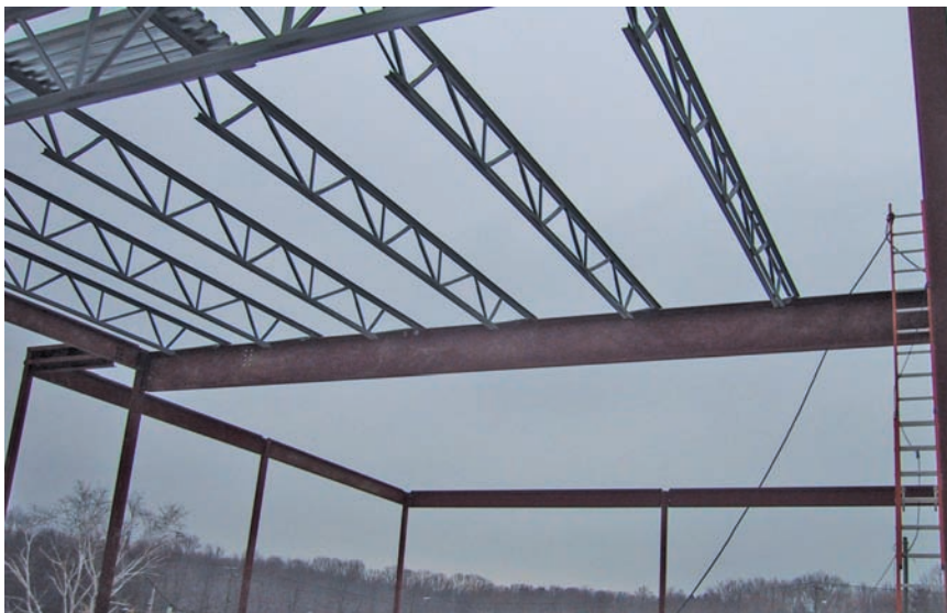
Photo 9.2 In this roof structure, each of the joists applies a concentrated load to the beam that supports it.
