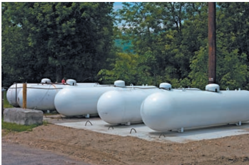
Photo 7.3 Cylindrical pressure vessels.
