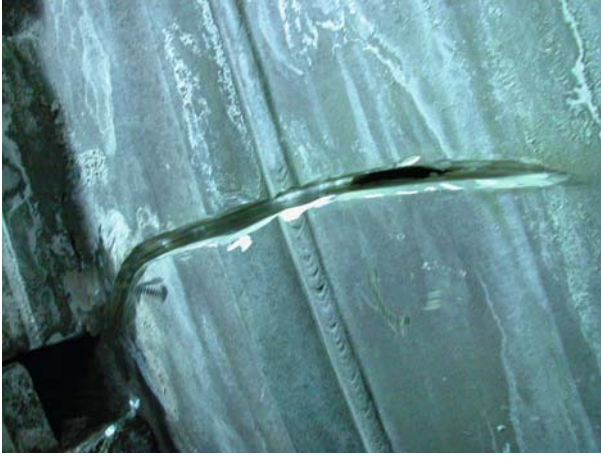
FIGURE 12.3 Thermal stress rupture of an 8.5 foot diameter tube used in a calciner, a device for treating liquid waste and turning it into high-level solid waste.
