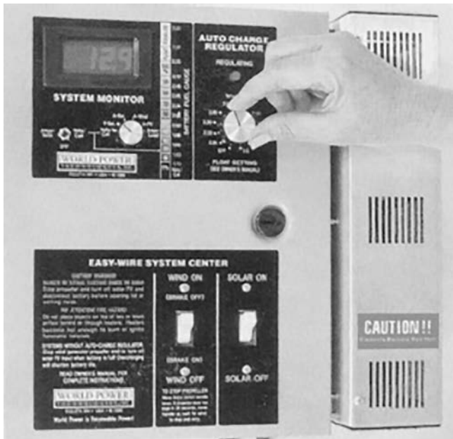
FIGURE 15.8 Integrated power connection and control unit for wind–PV–battery hybrid system. (From World Power Technologies, Duluth, MN. With permission.)
