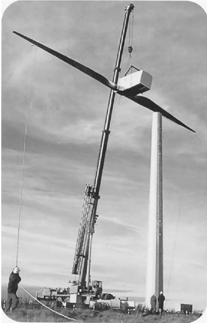
FIGURE 4.6 WEG MS-2 wind turbine installation at Myers Hill. (From Wind Energy Group, a Taylor Woodrow subsidiary and ETSU/DTI, U.K.)
