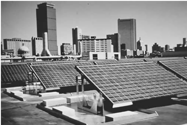
FIGURE 16.2 18 kW grid-connected PV system on the Northeastern University Student Center in Boston. (ASE Americas, Billerica, MA. With permission.)
